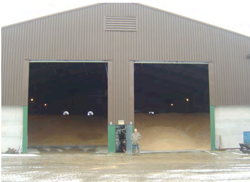
James Balaam with the 4,000 tonne store featuring Hydor Belt Drive HV fans in the bottom end of the store.
